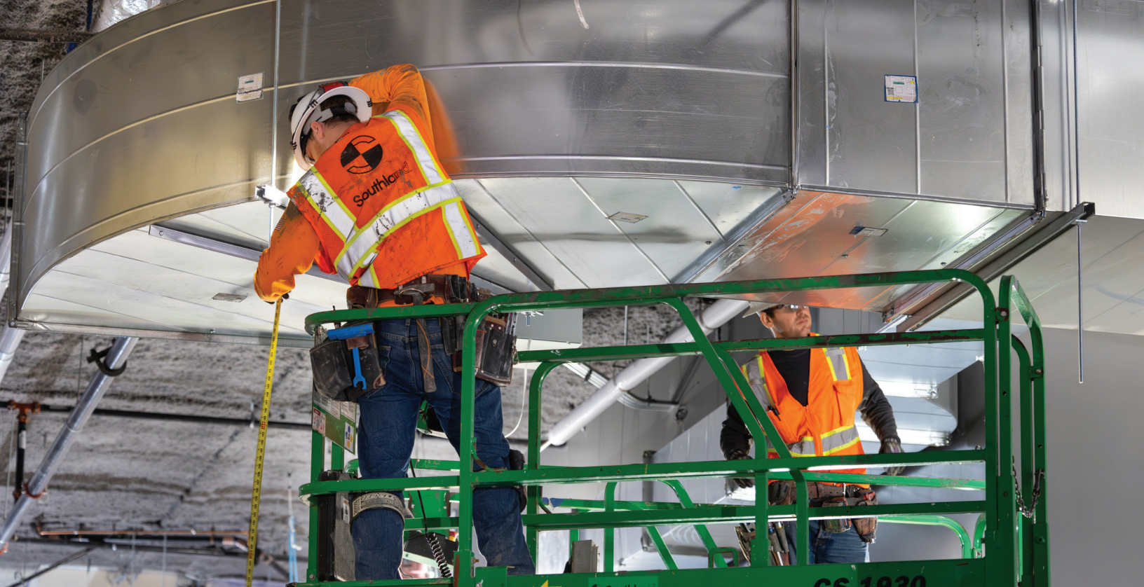
Southland workers installing duct at the Samuel Oschin Air and Space Center.
