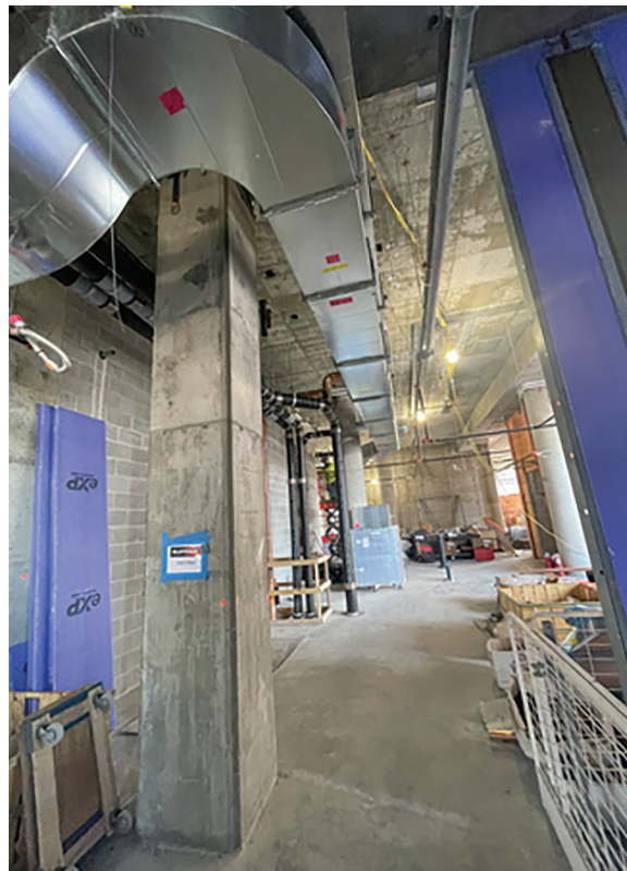
Left: Much of the ductwork for the hotel was manifolded at United HVAC's sheet metal shop before being installed on site. Right: Rectangular duct hangs in the hotel's second floor. The project used 107,000 pounds of ductwork.
