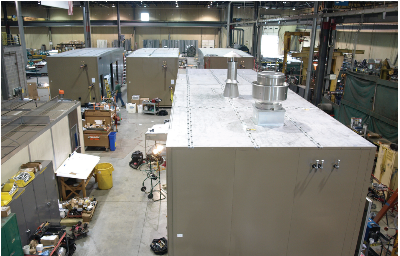
H.T. Lyons was involved in all of the mechanical aspects of these buildings — from sheet metal to piping to plumbing.
