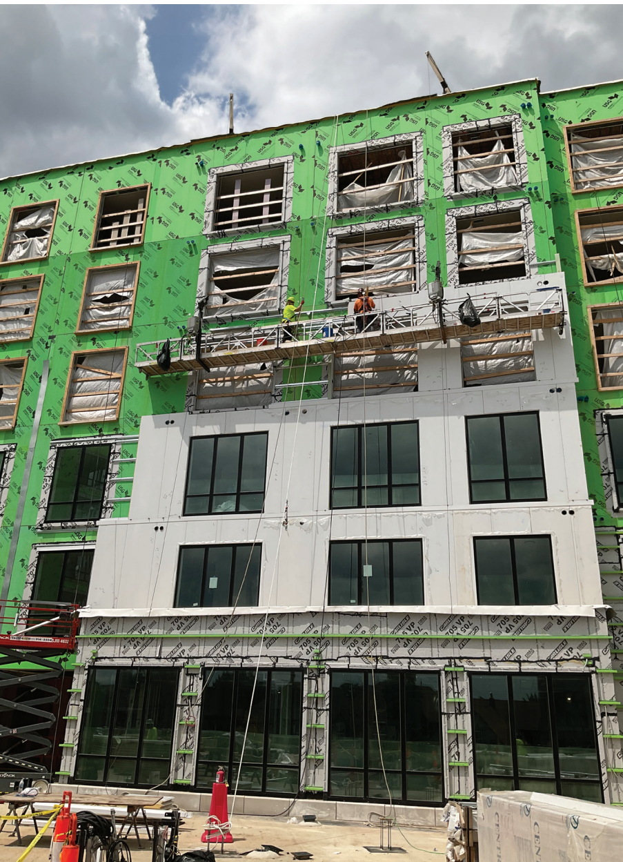
Perennial Corktown Apartments is a seven-story facility that includes 188 apartments and seven townhomes.
