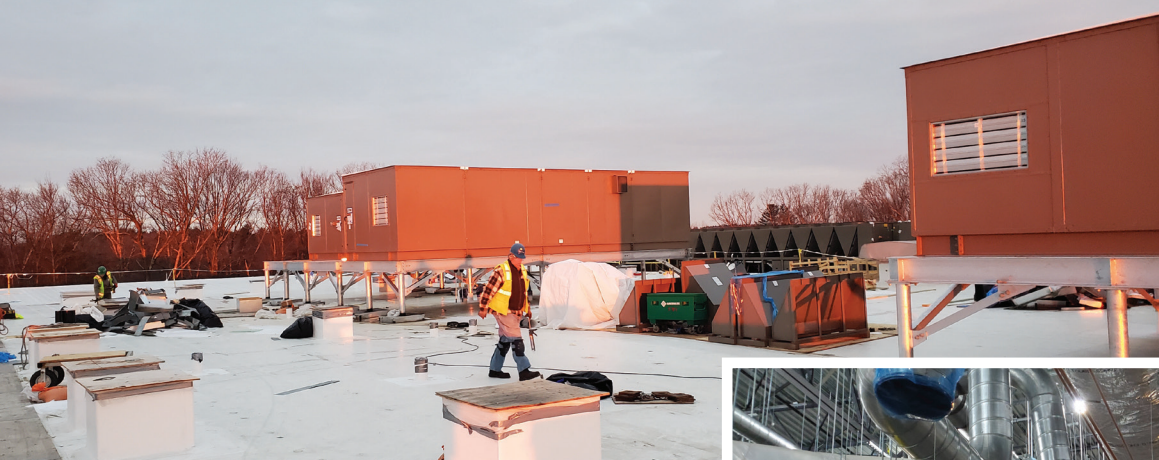
Left: Four air handlers on the Resilience building's roof were installed by United HVAC and union pipefitters. They range from 12,000 to 16,000 cubic feet per minute (CFM).
