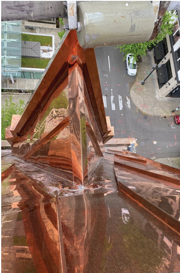
Project challenges included navigating a busy downtown environment while ensuring both public and employee safety.
