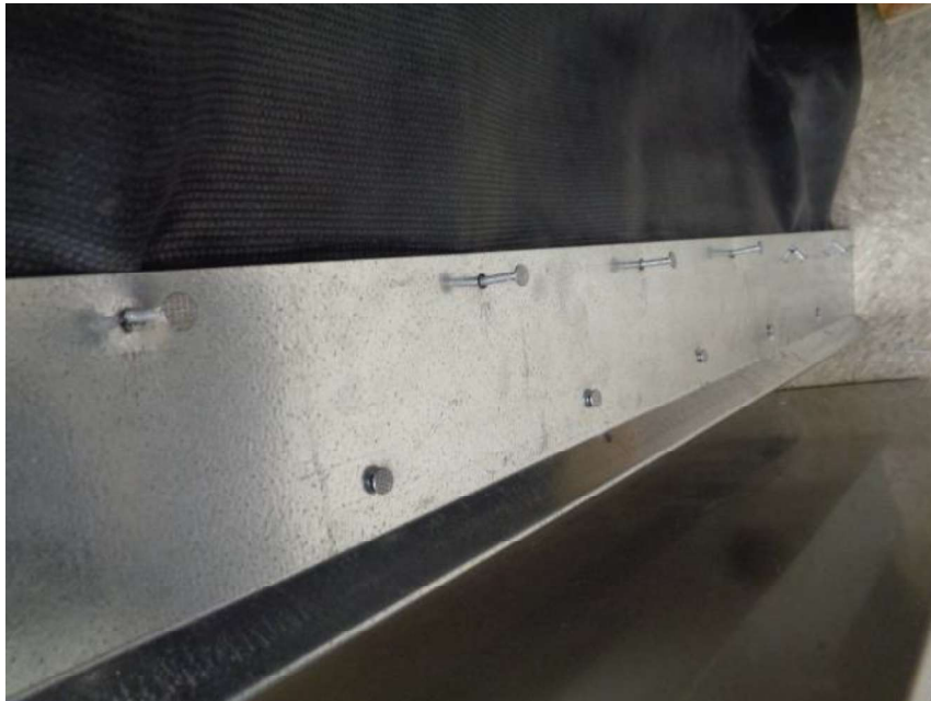
Photo No. 2 ANSI/SPRI Test RE-1 Typical Mode of Failure
