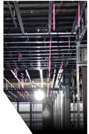
Because of logistical difficulties with the more than 100-year-old building, most of the 20,000 pounds of the metal used in the project had to be prefabricated and moved through the building's original elevators.
